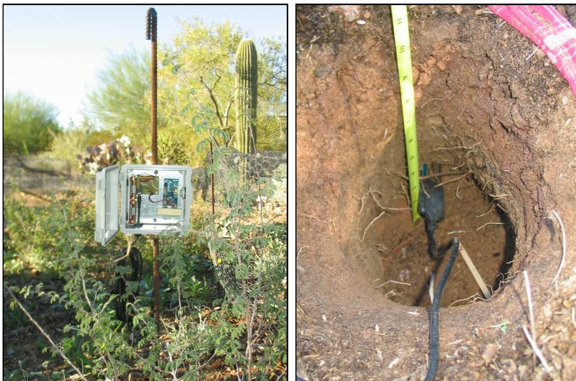
(a) Enclosure containing a Tmote wireless module and probe interface circuitry, installed in Bed 2.
